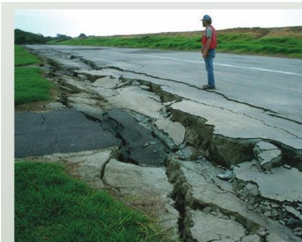
▶ DURING AN EARTHQUAKE IN CALIFORNIA, THE LAYER OF SAND UNDERLYING THIS HIGHWAY BECAME LIQUEFIED, CAUSING THE ROAD SURFACE TO CRACK INTO RUBBLE.
