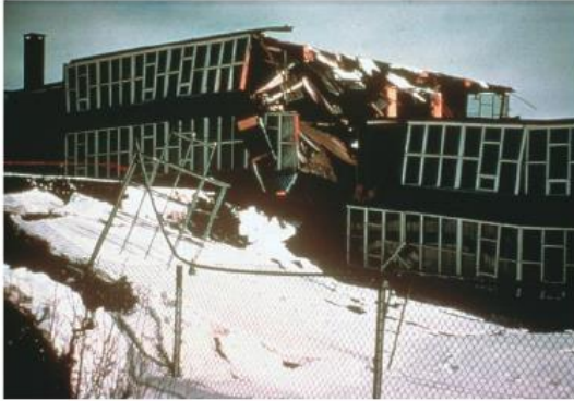
▶ THIS SCHOOL SPLIT IN HALF WHEN SOME OF THE SOIL UNDER IT MOVED DOWNSLOPE DURING THE EARTHQUAKE IN PRINCE WILLIAM SOUND, ALASKA.
