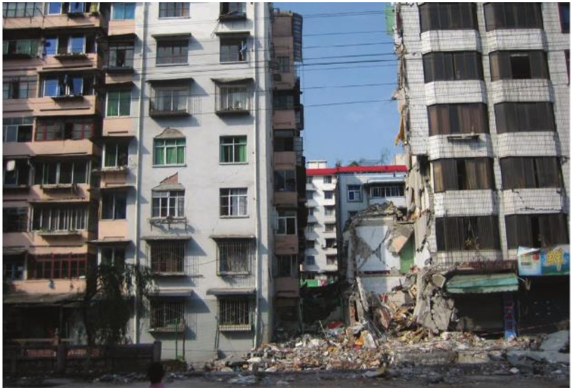
A 2008 EARTHQUAKE IN SICHUAN, CHINA, CAUSED A SECTION OF THIS BUILDING TO COLLAPSE.
