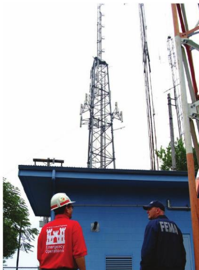
▶ AFTER A SERIES OF EARTHQUAKES IN 2006, ENGINEERS INSPECT A TRANSFORMER IN HAWAII TO MAKE SURE THAT IT REMAINS OPERATIONAL AT A SITE THAT TRANSMITS EMERGENCY MESSAGES.
