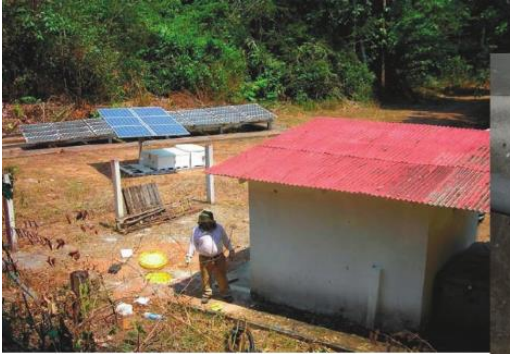
▶ SOLAR PANELS ARE USED TO POWER THIS SEISMIC MONITORING STATION IN THE BRAZILIAN AMAZON.
