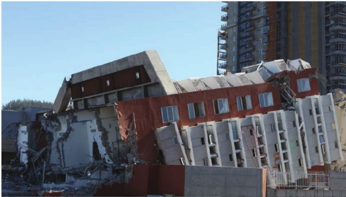
THIS APARTMENT BUILDING IN CONCEPCIÓN, CHILE, COLLAPSED AS A RESULT OF AN EARTHQUAKE IN FEBRUARY 2010.
